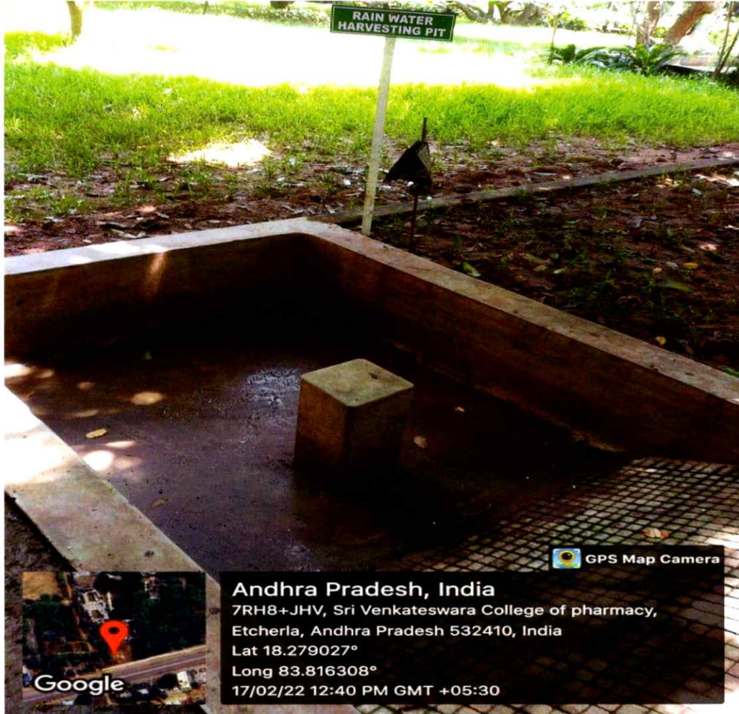
Rainwater Harvesting Pit
